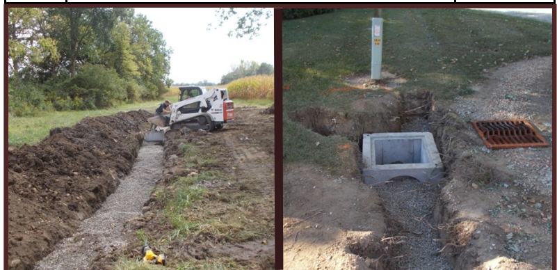
The upper left picture is an example of a sectional tile main replacement. To the right is a catch basin and lateral repair. Both projects were completed in 2025.
